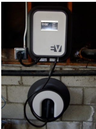
Sedan's charger, in garage.
