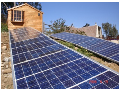
Our PV 2 added 2.8 kW more power to total 6.5 kW solar overall.
