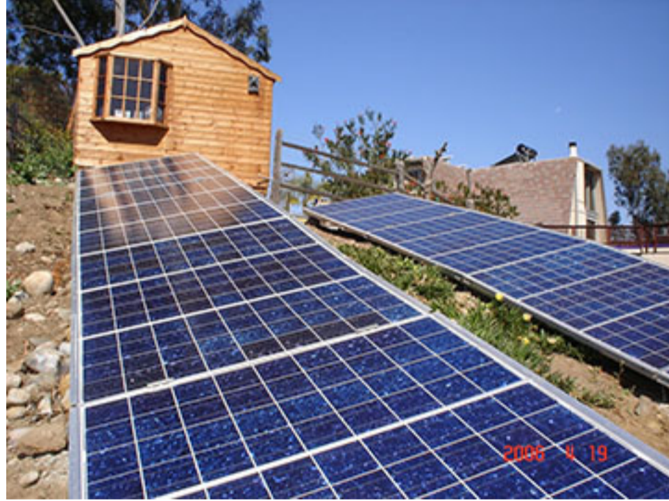
Ground mounted poly PV.
